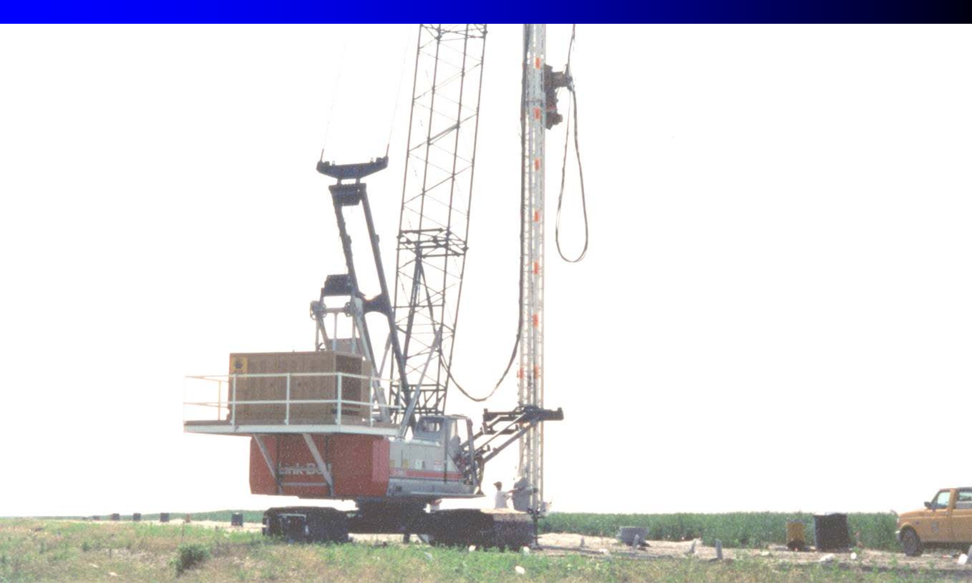
APE top mounted Model 50 fitted with 170 feet of APE ST 75 leads mounted on Link belt crane at Craney Island
