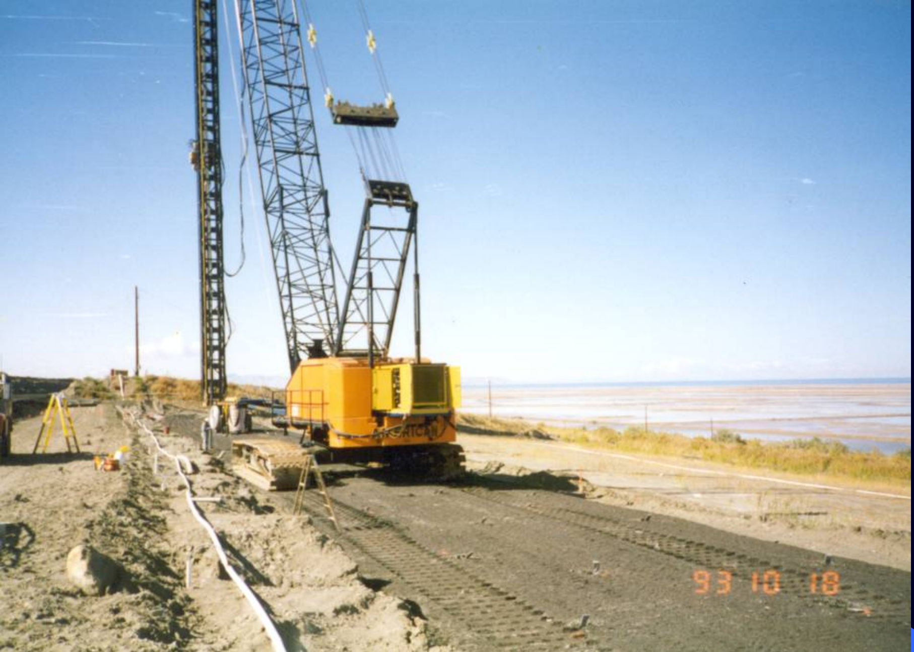
Another view of APE equipment in Salt Lake. Top drive vibro only. Note that APE power unit is mounted on back of 300 ton crane.
